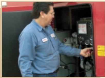
Doors allow easy access to operating controls.
