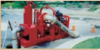
8NCRD 8" non-clog pump used on a bypass site in Freeport, IL.
