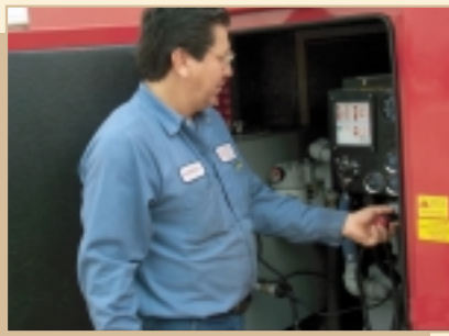
Doors allow easy access to operating controls.
